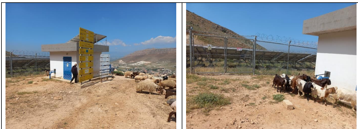
Figure 1.1: Kfarzabad solar water pumping station
