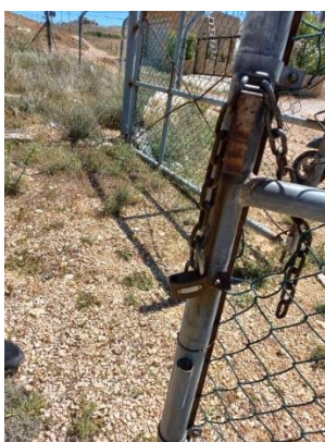
Figure 3.5: Damaged fence padlock
