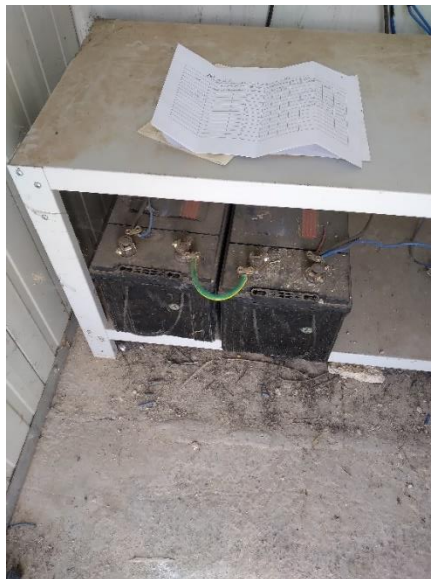
Figure 2.2: Existing 2 lead acid batteries
