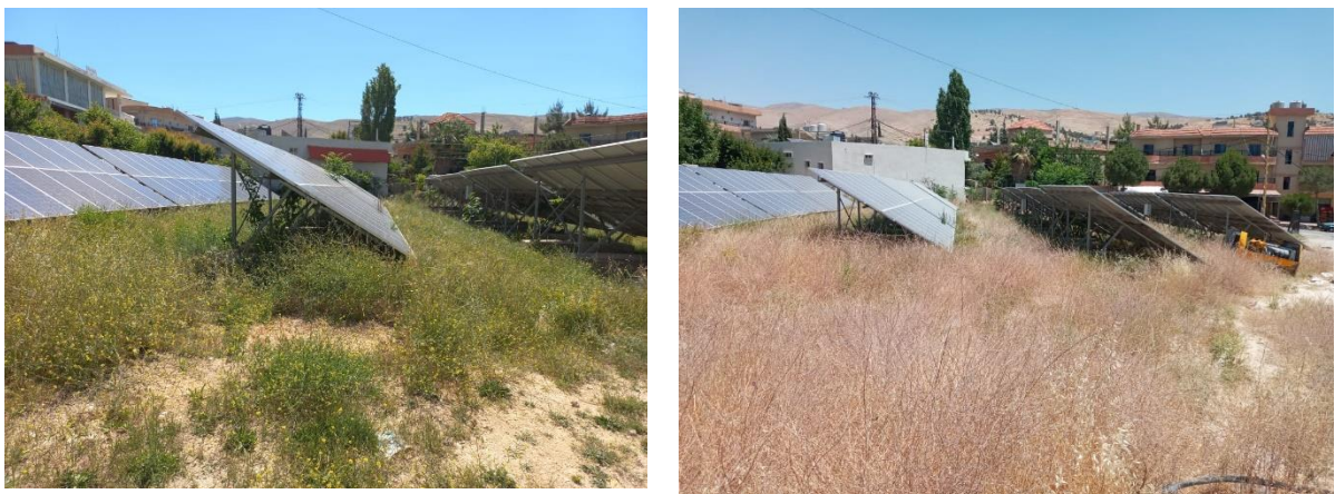
Figure 2.4: Grass under and around the PV panels in May 2024 (left) and Summer 2023 (right)
