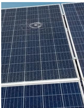
Figure 2.3: Broken PV panel (hit by a bullet)
