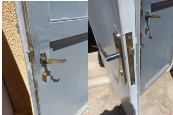
Figure 5.1: Door locks needs to be replaced or maintained.
