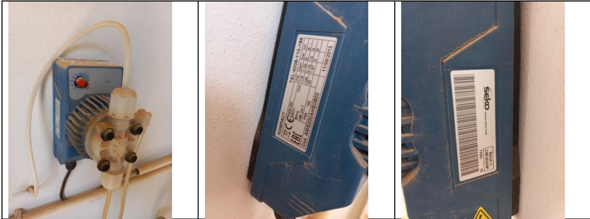
Figure 1.2: Chlorination system pump
