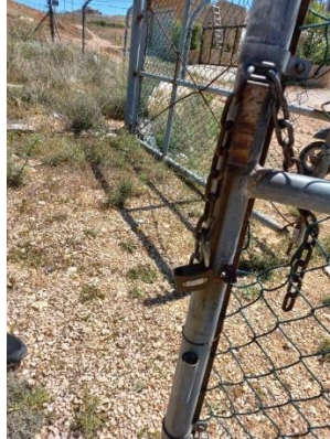
Figure 3.4: Damaged fence padlock
