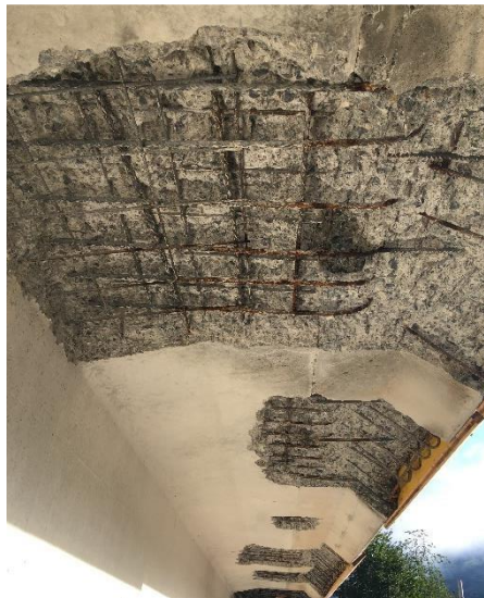
Figure 1. Substrate preparation by concrete removal with high water pressure and placing of formwork (right)
