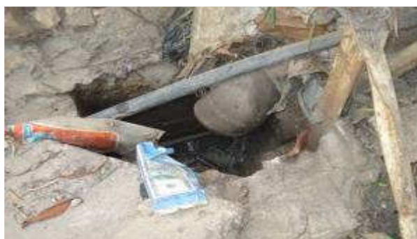
Damaged manhole crossed by water supply pipe
