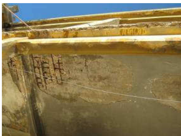
Damaged concrete floor
