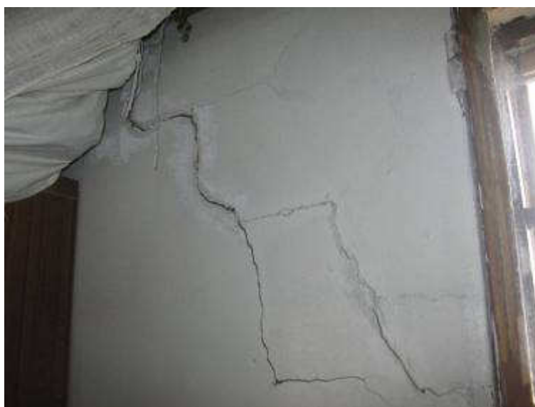
Diagonal crack in masonry (symptomatic of major structural problem)
