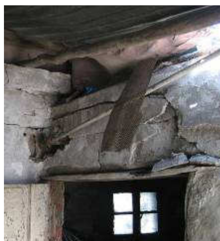
Cracked concrete lintel
