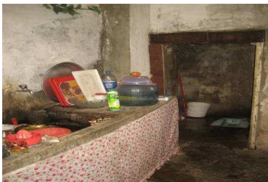
Kitchen and bathroom affected by high humidity and missing separation
