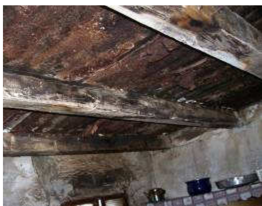
Old rusted zinc roof
