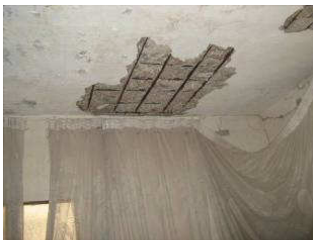
Damaged concrete roof, rusting reinforcements
