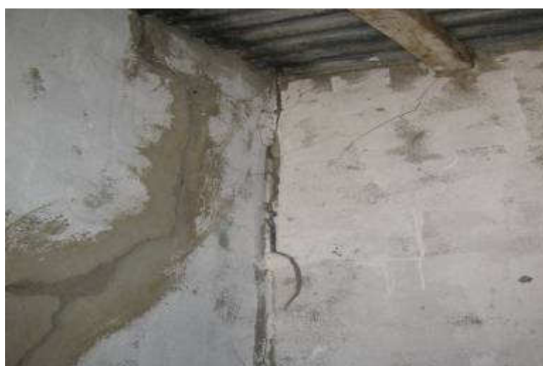
Crack in masonry
