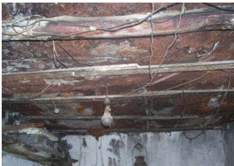
Outdated zinc roof
