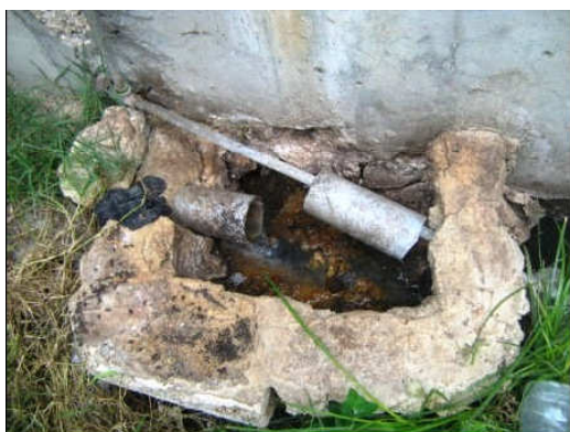
Open-air inspection chamber
