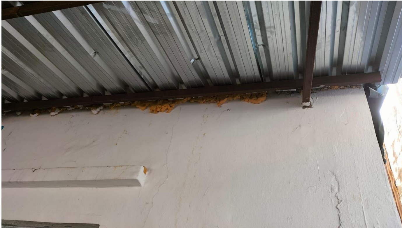
Photo 3-Missing Waterproofing (foam) between wall and Zinc in different areas
