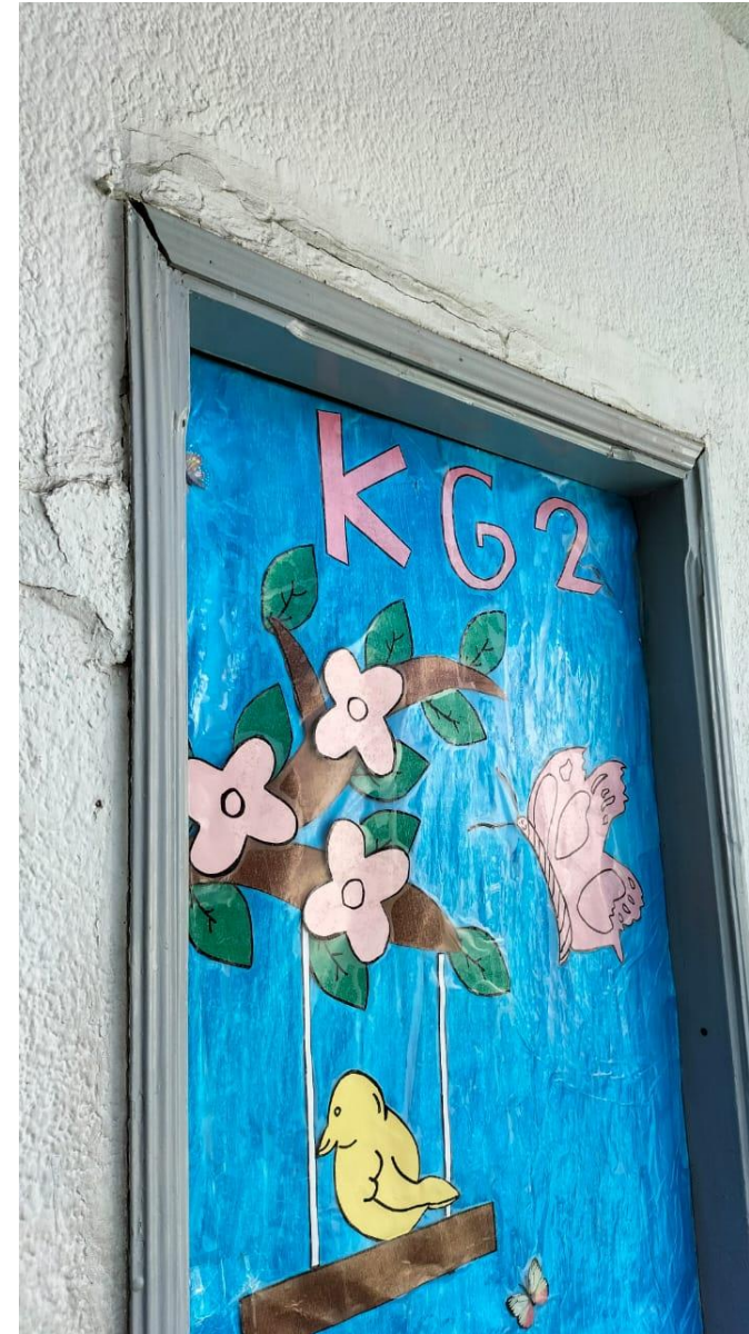
Photo 5-Damaged doors (can't be closed )
