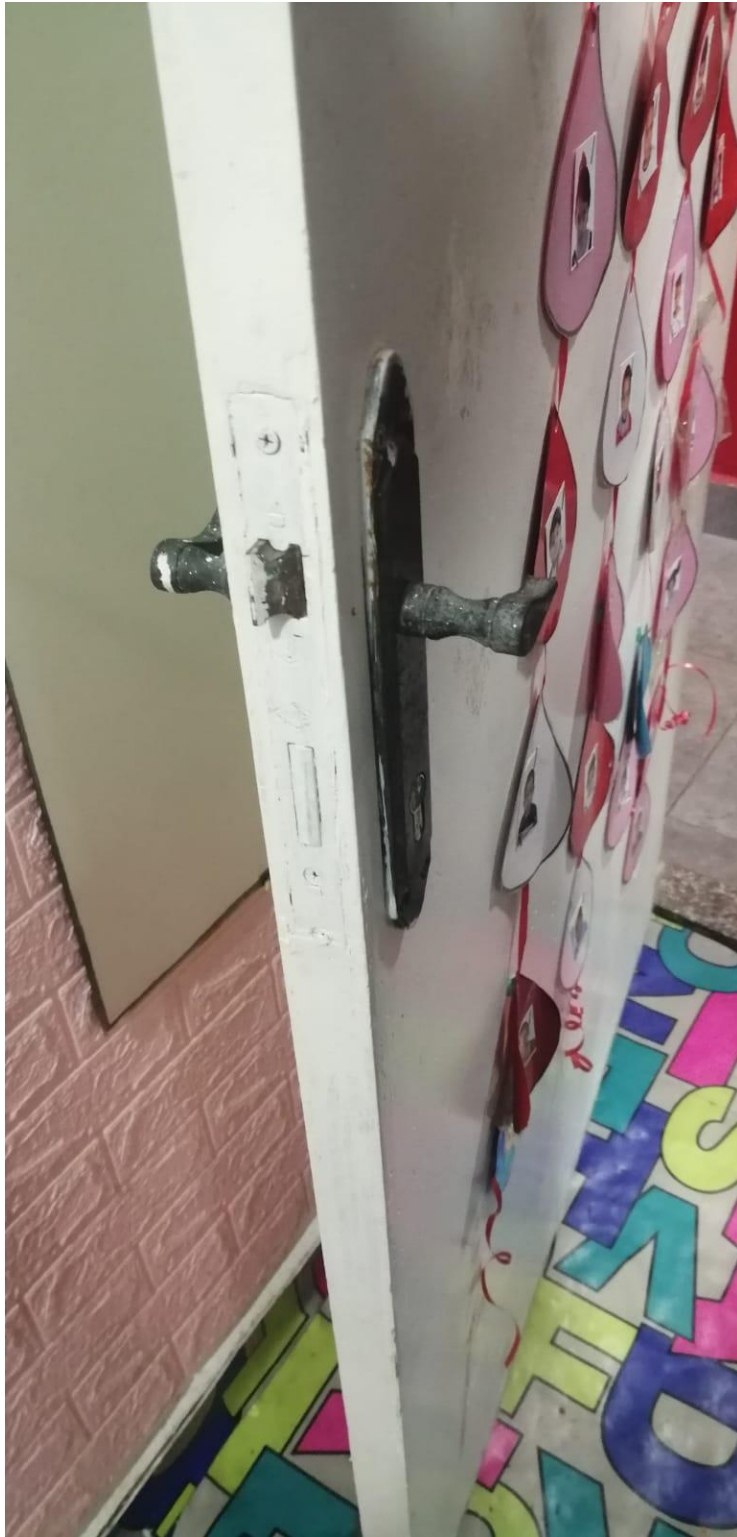
Photo 3-Door handle rusted and damaged
