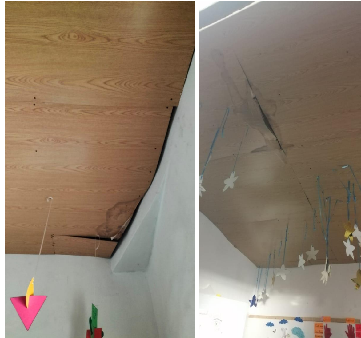
Photo 1.2- Water leakage from the ceiling
