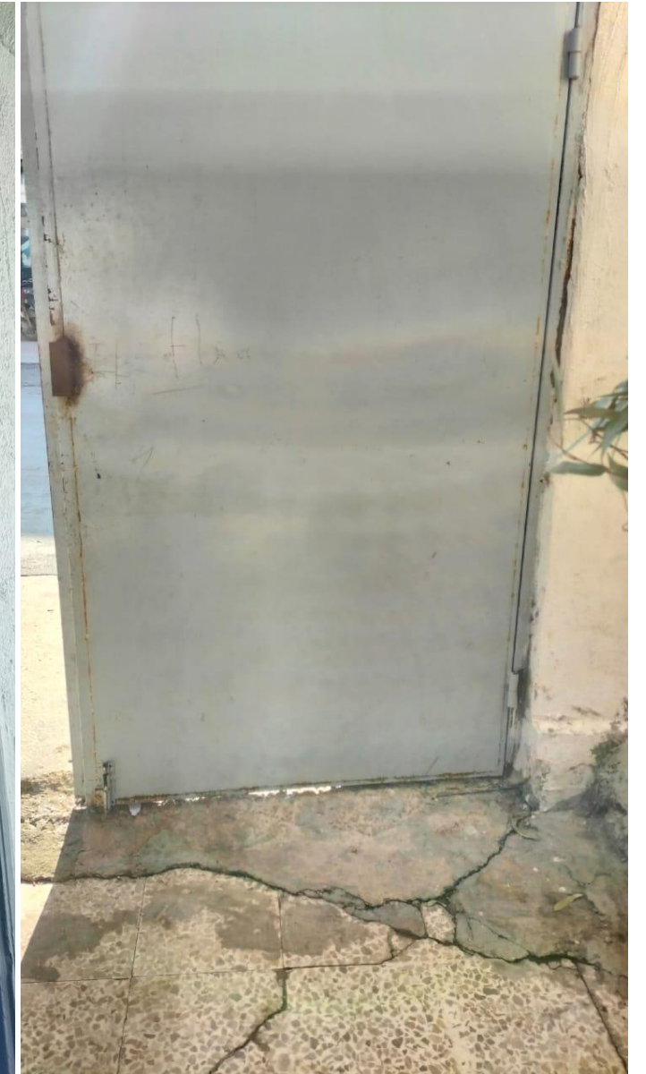
Photo 6- Entrance ramp cracks
