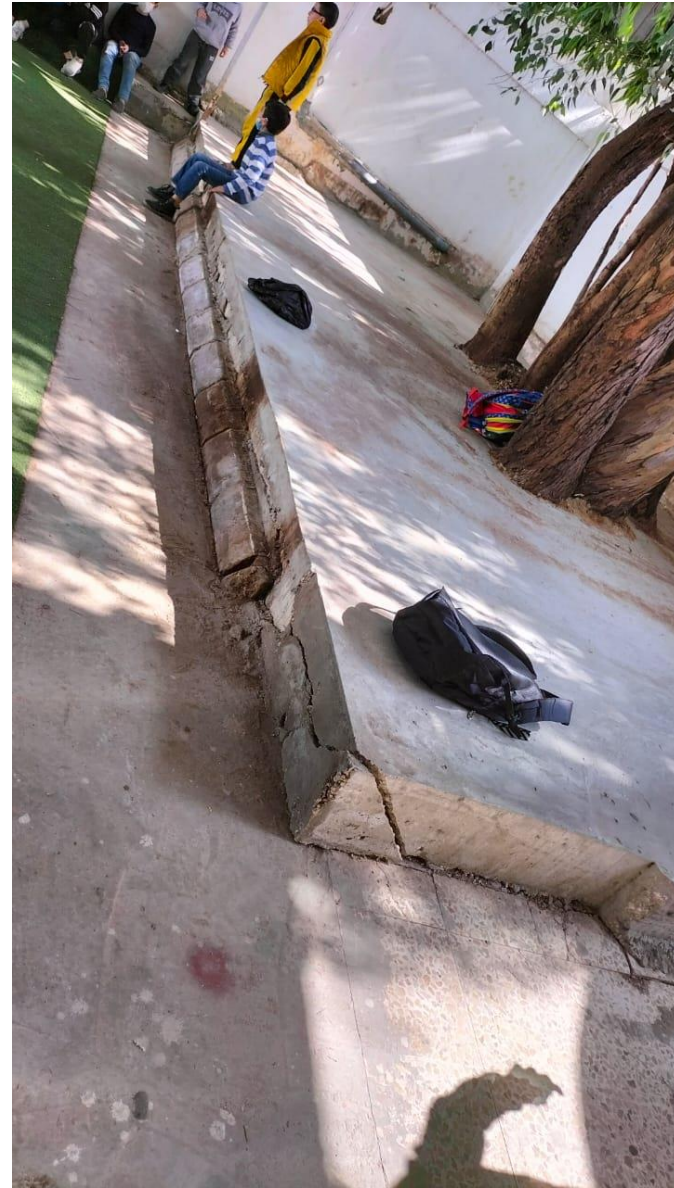
Photo 4-Cracks and unsafe parapets
