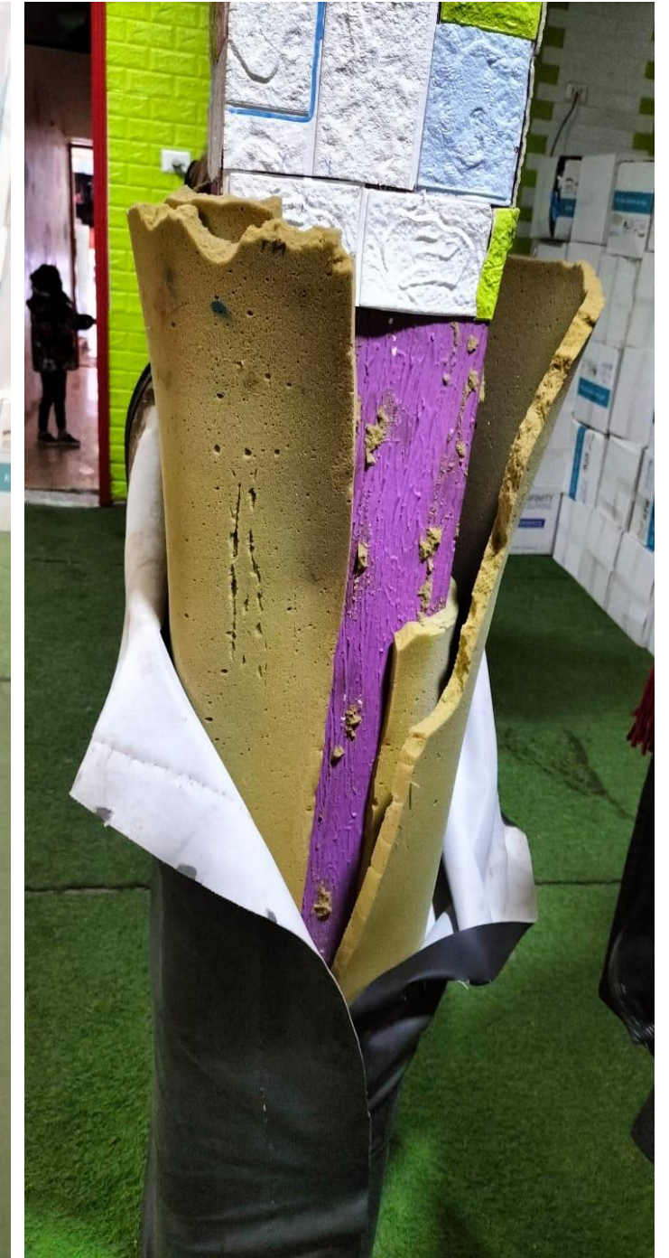
Photo 2- Column protection damaged
