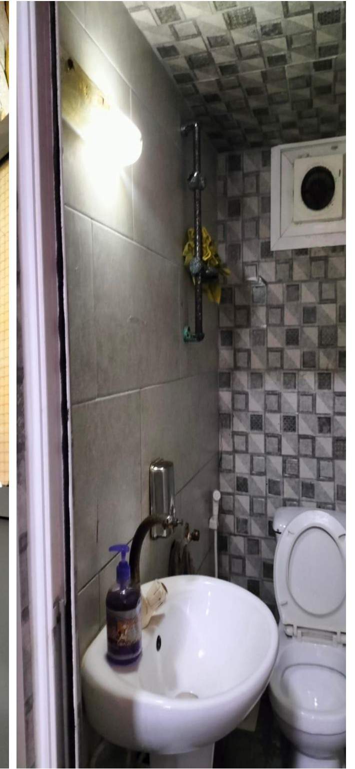
Photo 6- Damaged water faucet
