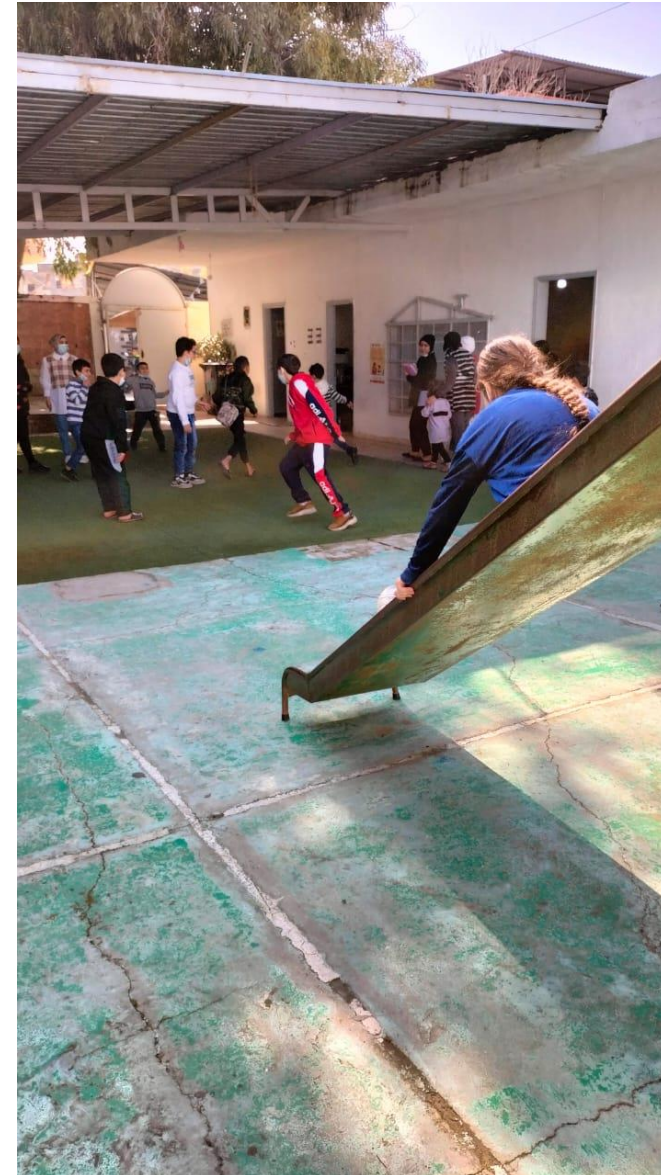
Photo 1- Play area (missing grass/soil treatment)
