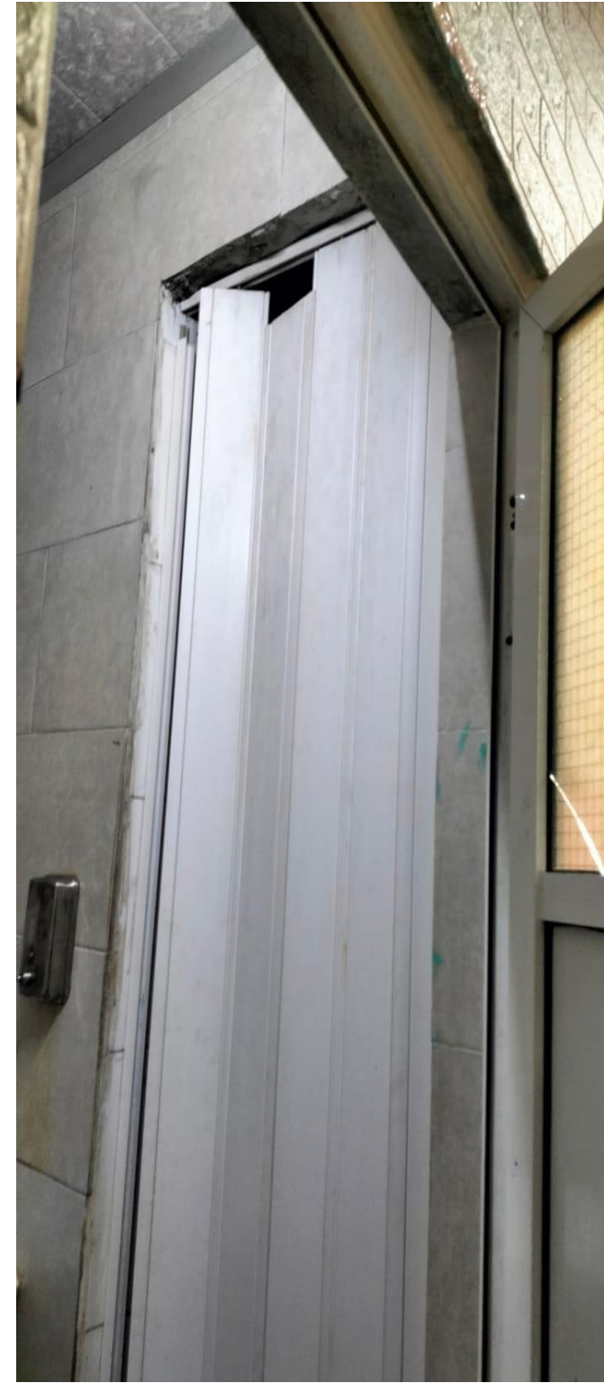
Photo 5- Damaged accordion door
