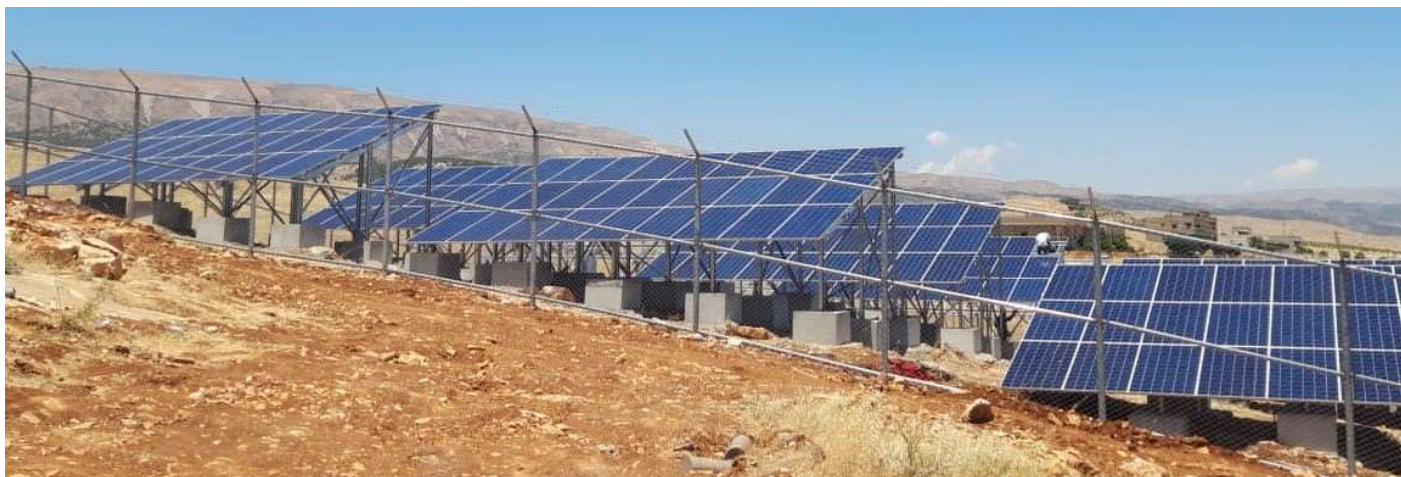
The photovoltaic systems provided by Switzerland to water pumping stations in the Bekaa.
