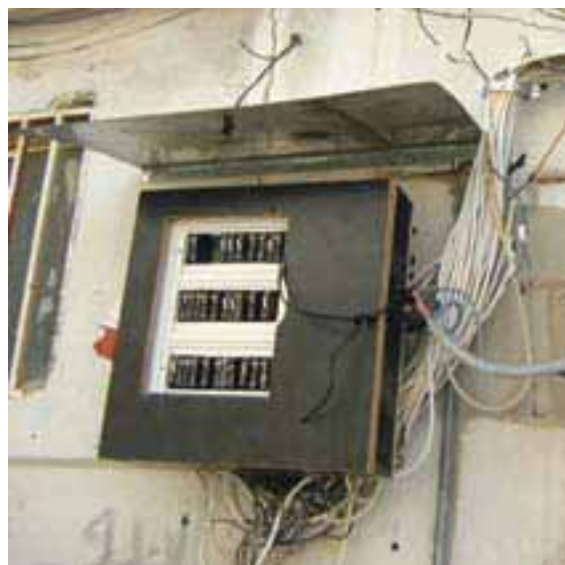
An example of organized electricity provision by the local committee in Fadlo Wakim AA around Ain el Helwe Camp (compare to unorganized electricity provision on p.63)
