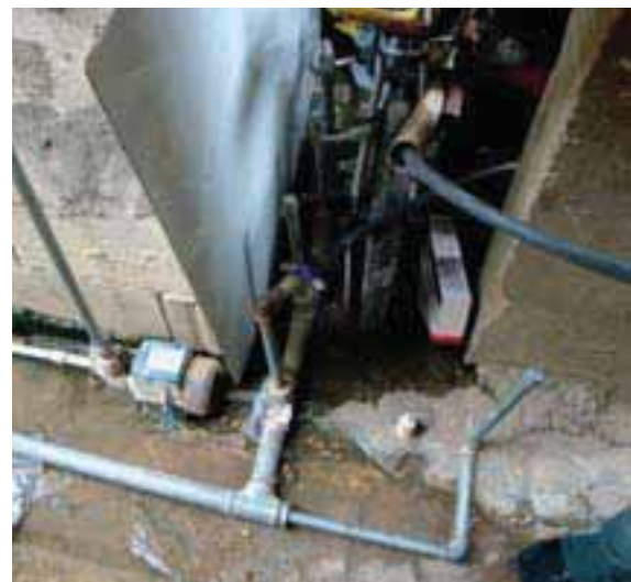
Water in Sekke is directly distributed from the well to single house connections
