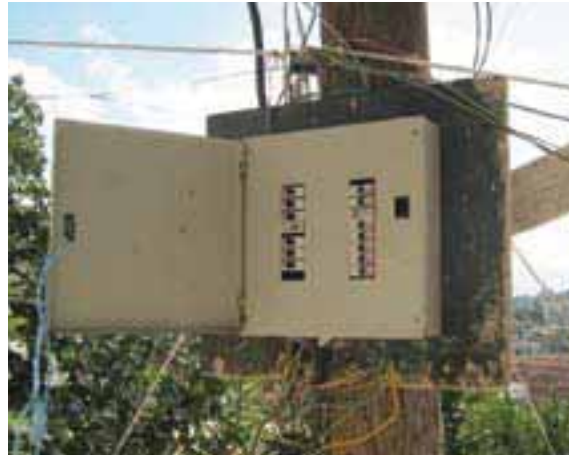
Electric distribution board installed by the Camp PC to organize electricity provision in Mieh Mieh AA
