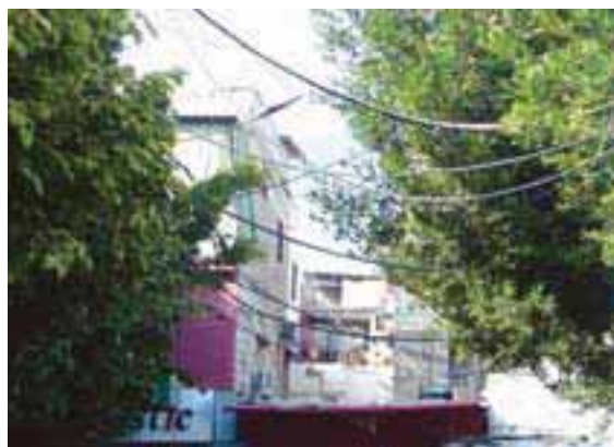
Water provision in Hay el Sohoun is compromised by the ad-hoc electricity connections (Note partially repaired cables)
