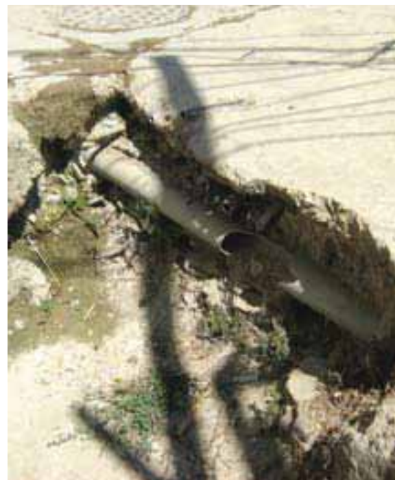
Broken sewage pipes in Mieh Mieh AA
