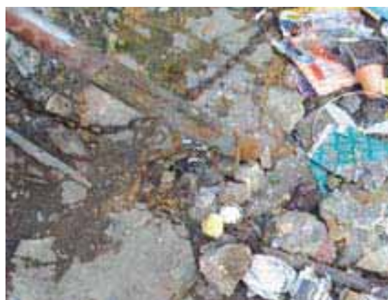
Partially exposed networks in Hay el Sohoun cause potential water contamination by sewage
