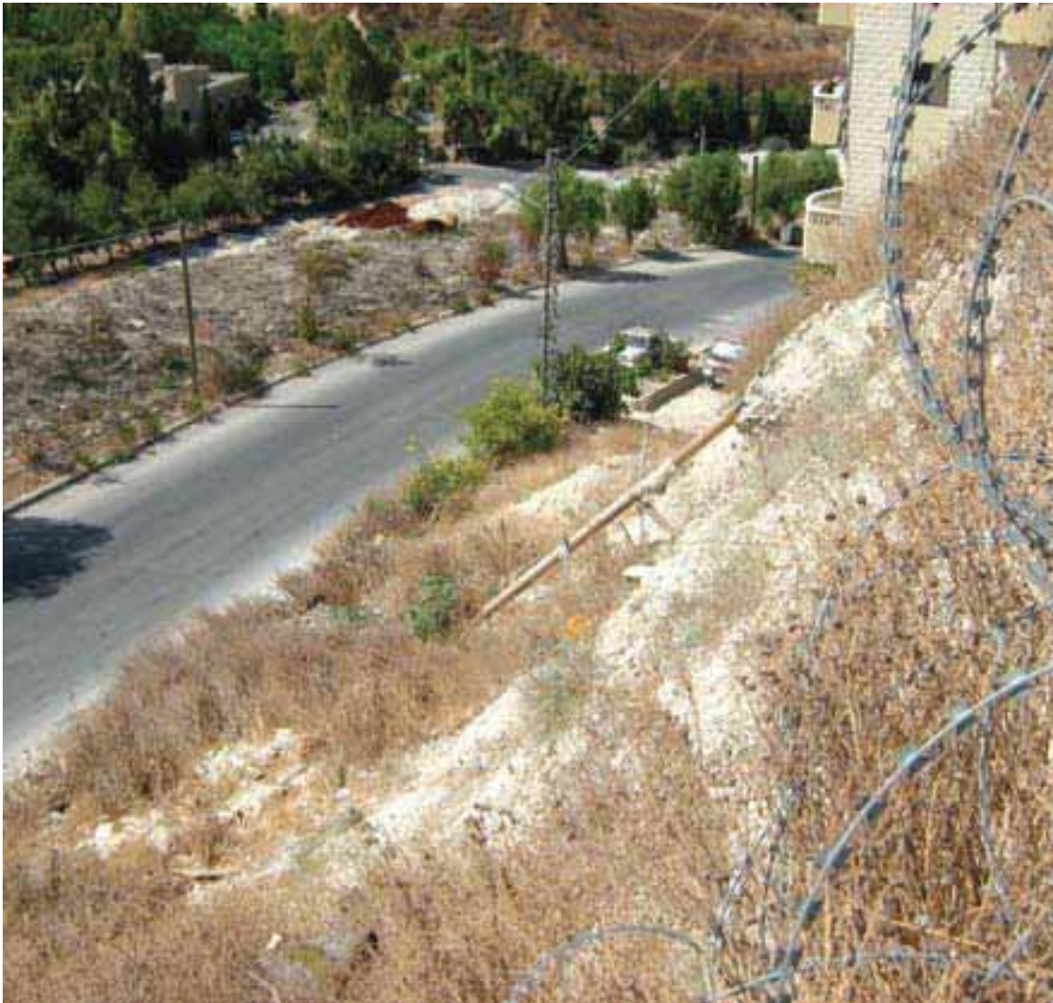
A sewage pipe discharging without proper connection from Hay el Wadi in Mieh Mieh AA to the surrounding Mieh Mieh village in South Lebanon
