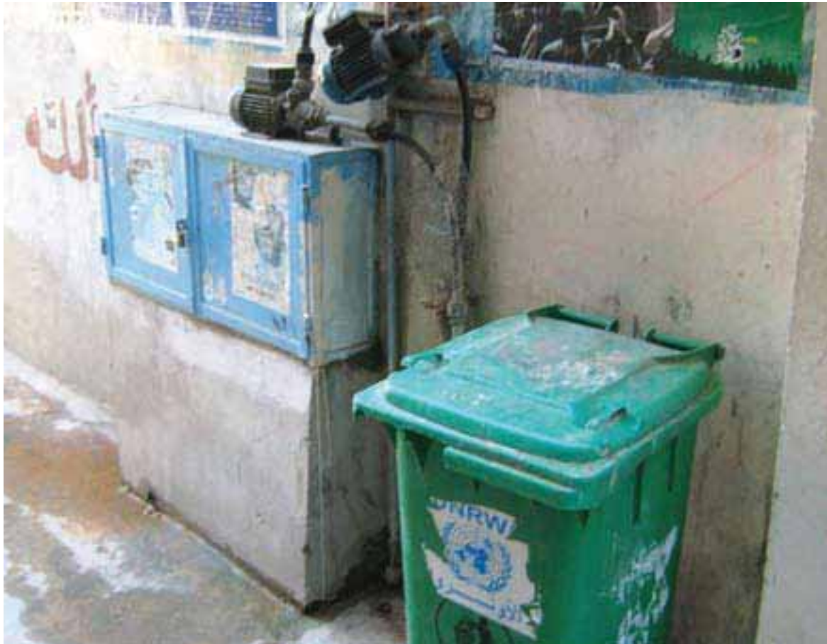
UNRWA informally extends some BUS to the AAs, note the collective water manifold and the solid waste container in the AA of Mieh Mieh Camp
