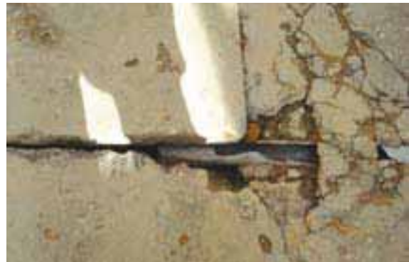
Damaged sewage pipes in Bustan el Kods
