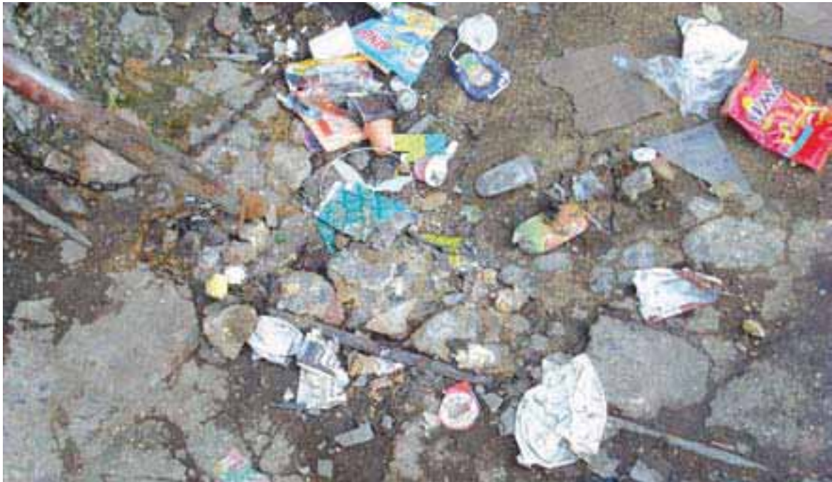
Most roads in Hay el Sohoun are in need of rehabilitation and asphaltting, taking into consideration the condition of the existing infrastructure networks
