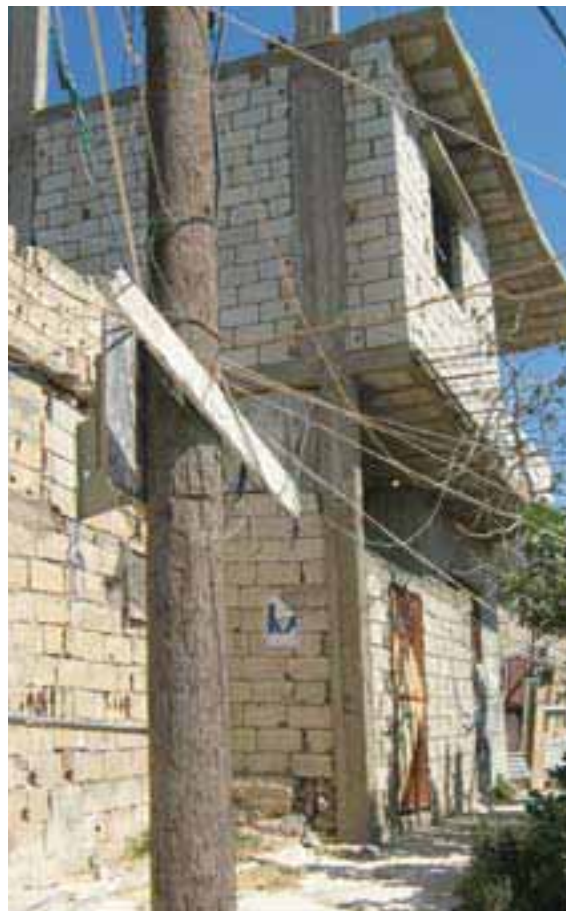
Basic methods for retaining loose and unshielded electricity cables in Hay el Wadi, Mieh Mieh AA
