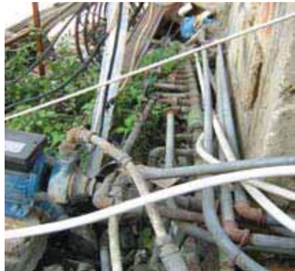
Direct implementation of water networks by dwellers in the AA of Jabal el Halib around Ain el Helwe Camp
