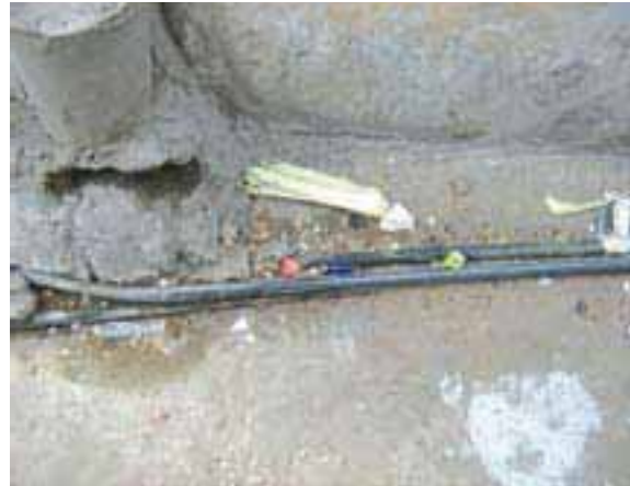
Above ground house connections installed by dwellers in Tawari to access water
