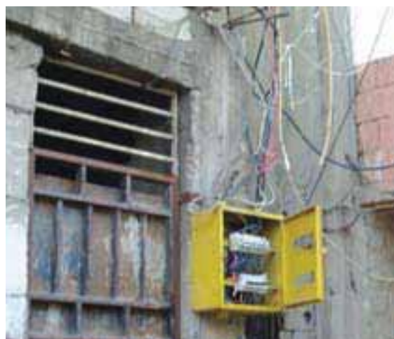
Electricity meters initially installed by EDL were replaced with direct connections to electric distribution boards by the SC in Hay el Sohoun
