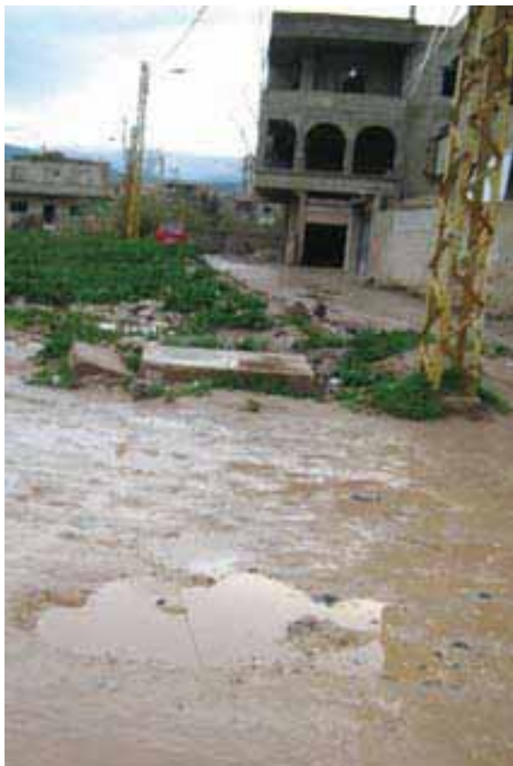
The unpaved roads covering the oil-pipe and the railway in NBC AA
