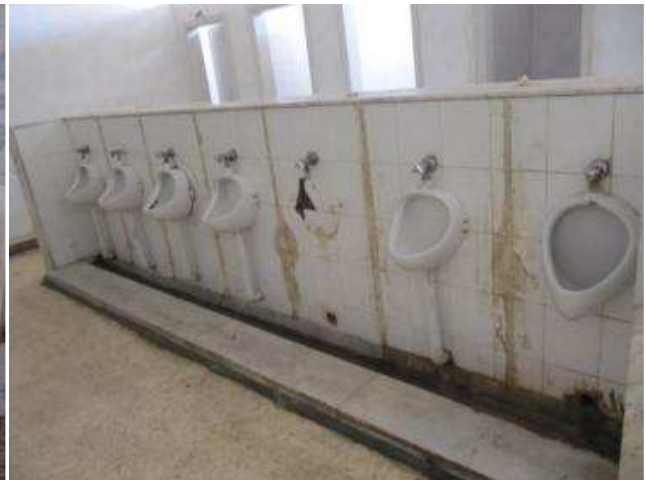
Urinals to be maintained
