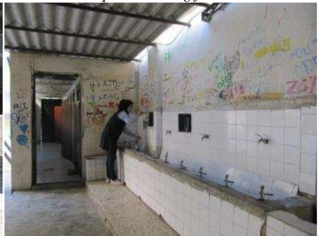
Drinking facility to be maintained
