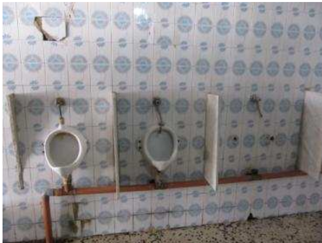
Urinals to be maintained
